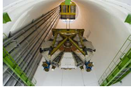
(b) Lowering of the SW in one of the two the access shafts to UX15.
